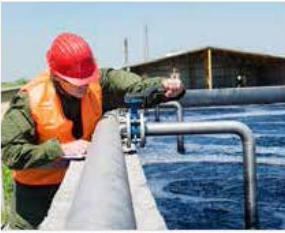
Wastewater Treatment Facility
