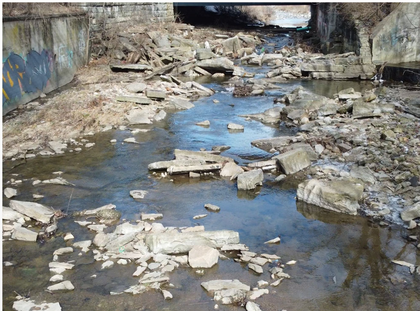
Debris from dam
